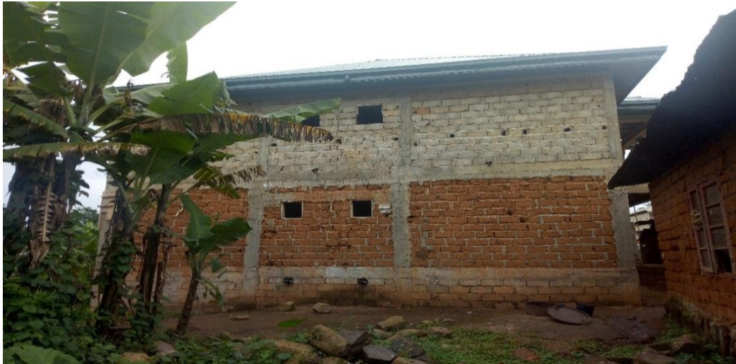
Figure 2: Showing a Blend between a Cement Block and Sundry in a G-Plus 1, around Foncha Street Source: (Ngala, 26 September 2021).
